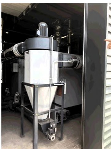
12-07-2022- sensor in rookgasafvoer ketel 2
